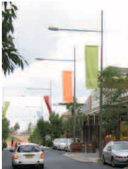
- Street Lighting – Rouse Hill Town Centre
