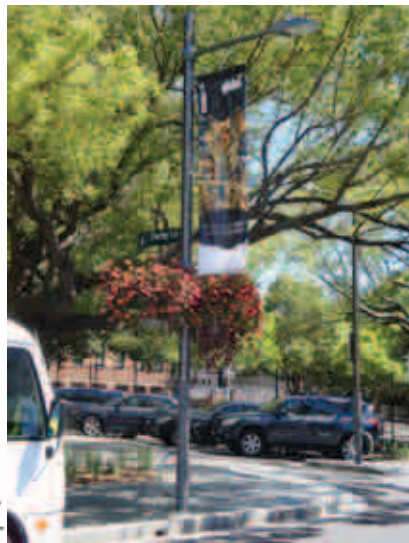
- Street Lighting – Glebe Point Road, Glebe
